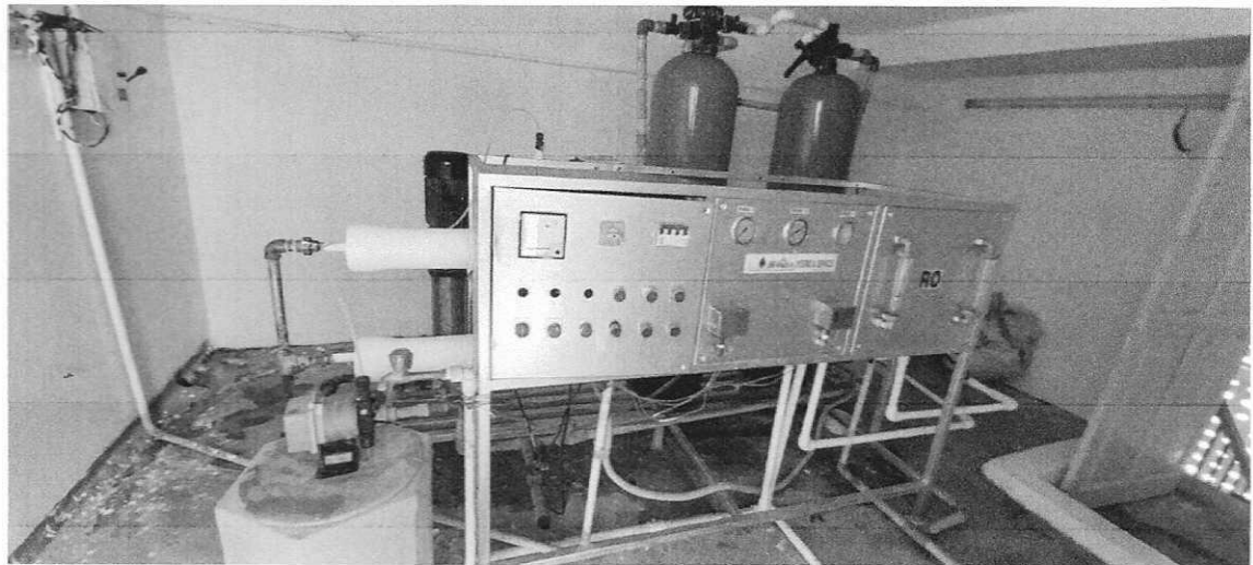
RO Plant Inside the Campus
