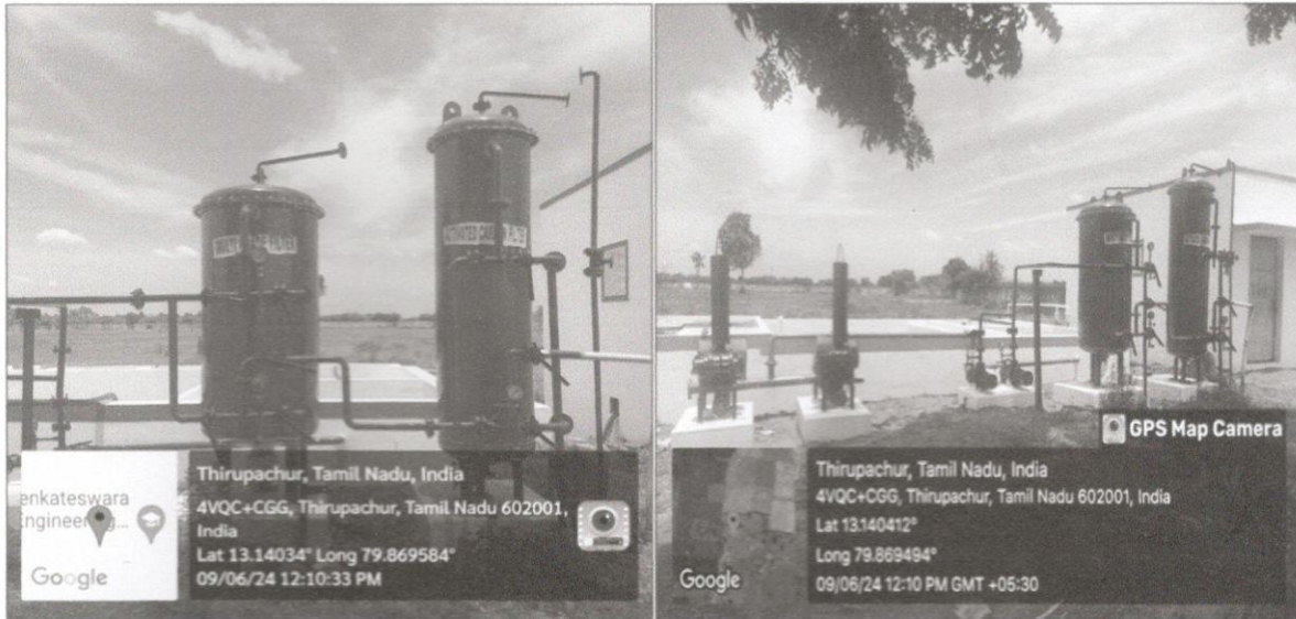
Waste water recycling system present in SVCET sports ground
