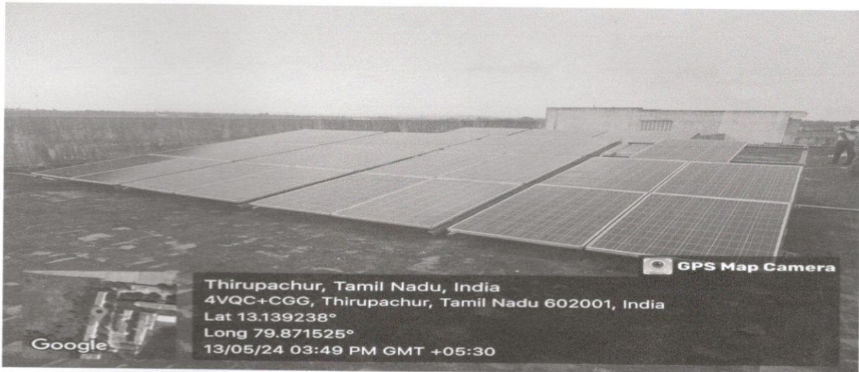
Solar energy panel installed at F-block (SVCET)
