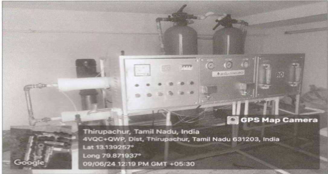
The RO Plant in B-block at SVCET
