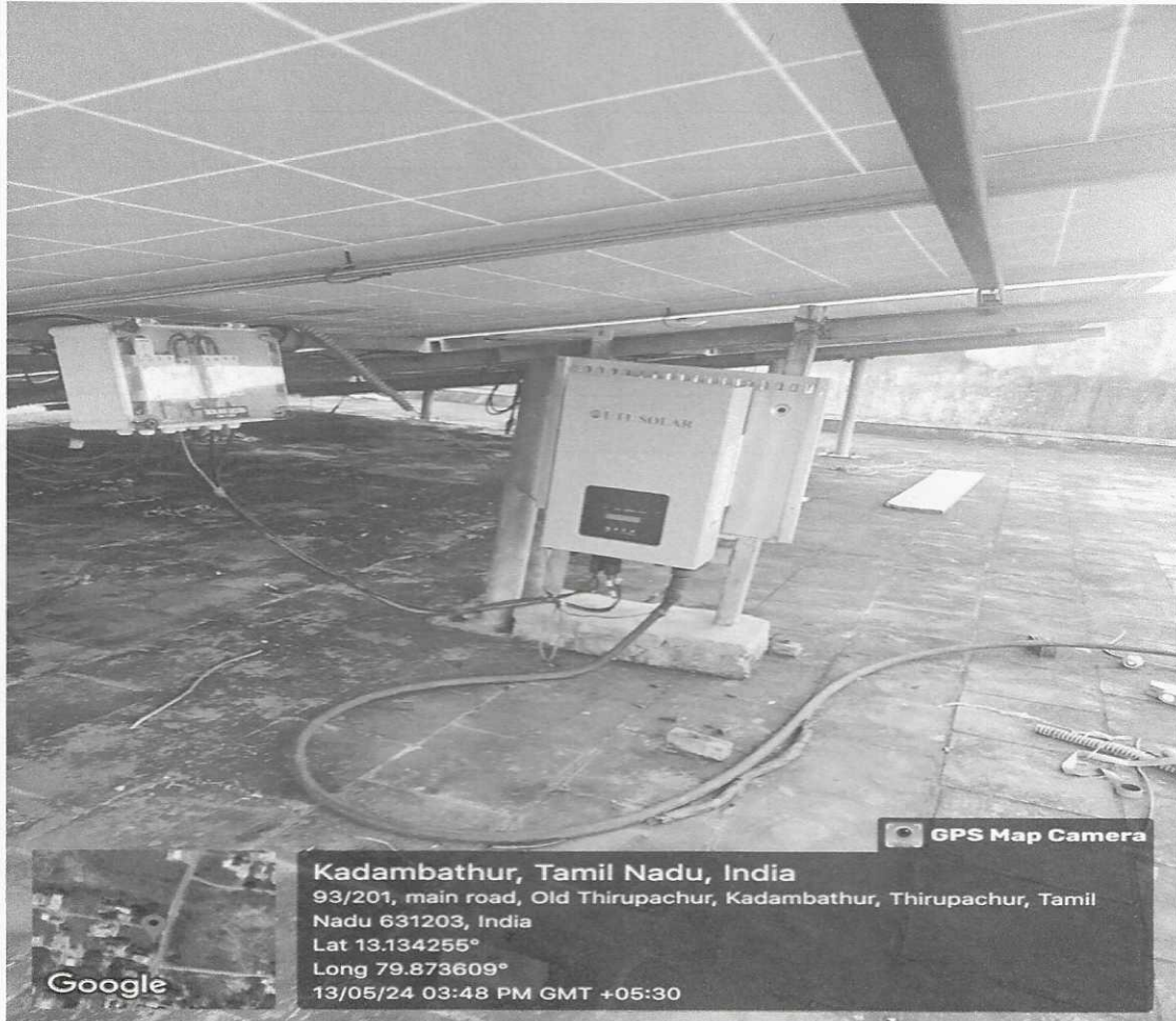
UTL solar installed at F-black ground floor
